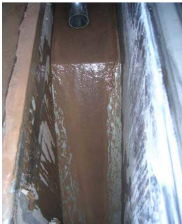
SCARICO FANGO SLUDGE OUTLET
